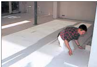
Installation of heat and sound insulation on a sufficiently load bearing and level substrate
